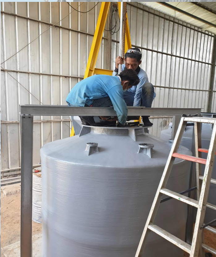
HDPE/FRP Urea Water Tank
