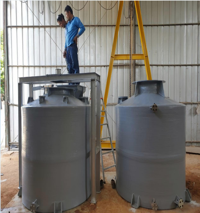
HDPE/FRP Urea Mixing Tank
